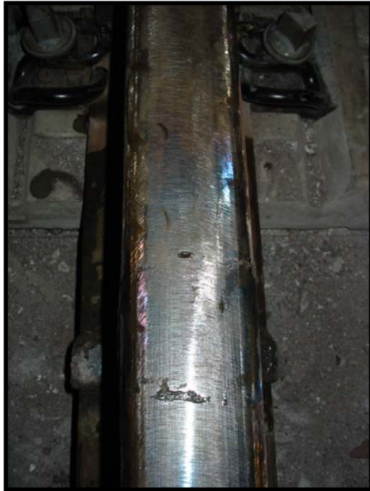
Figure 3 Sand burns on ground rail surface
