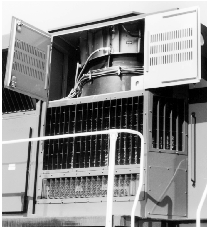
Figure 5 Typical Dynamic Brake Resistors, Fan, And Motor Application in 80, and 90 Series Locomotive Superstructure
