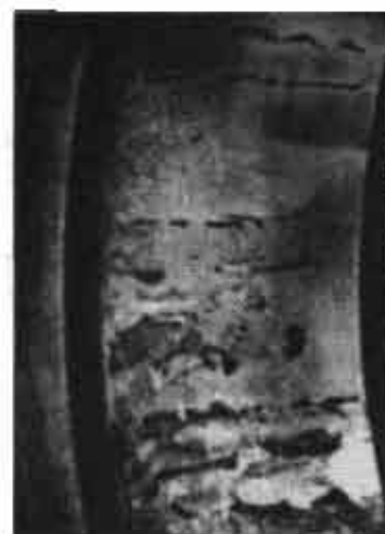
Corrosion, Pitting And Rust
